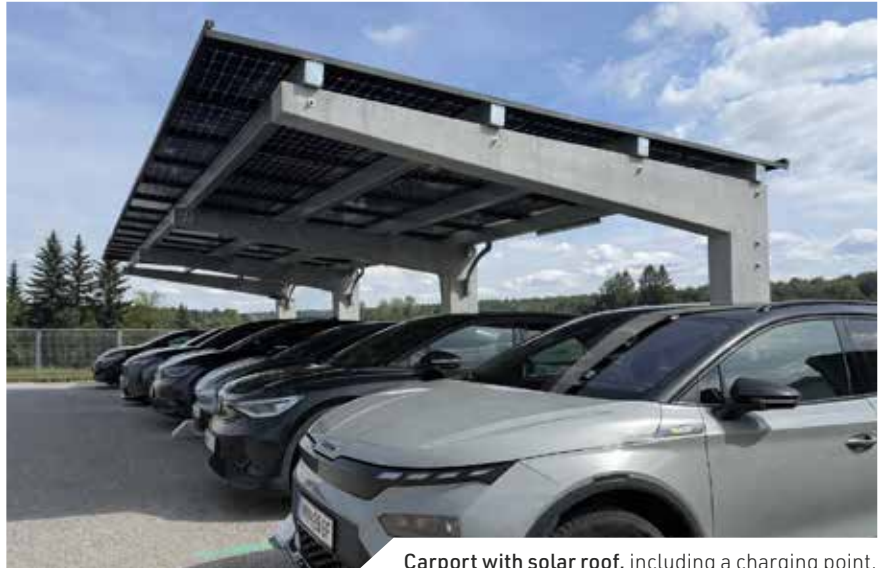
Carport with solar roof, including a charging point.
