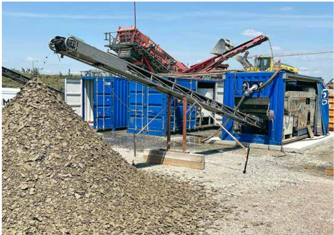
Disposal of the water drained sludge and possible reuse of the filter cake
