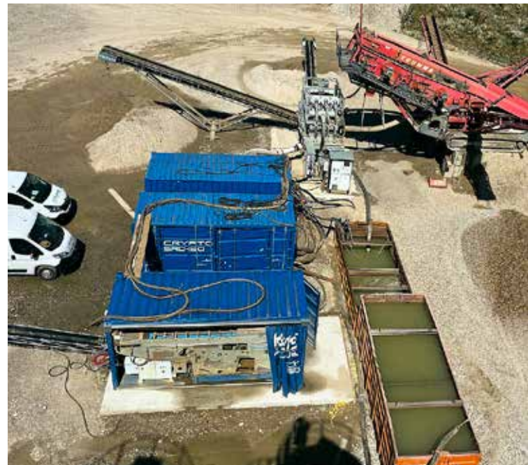
Containerised washing screen system and process water treatment
