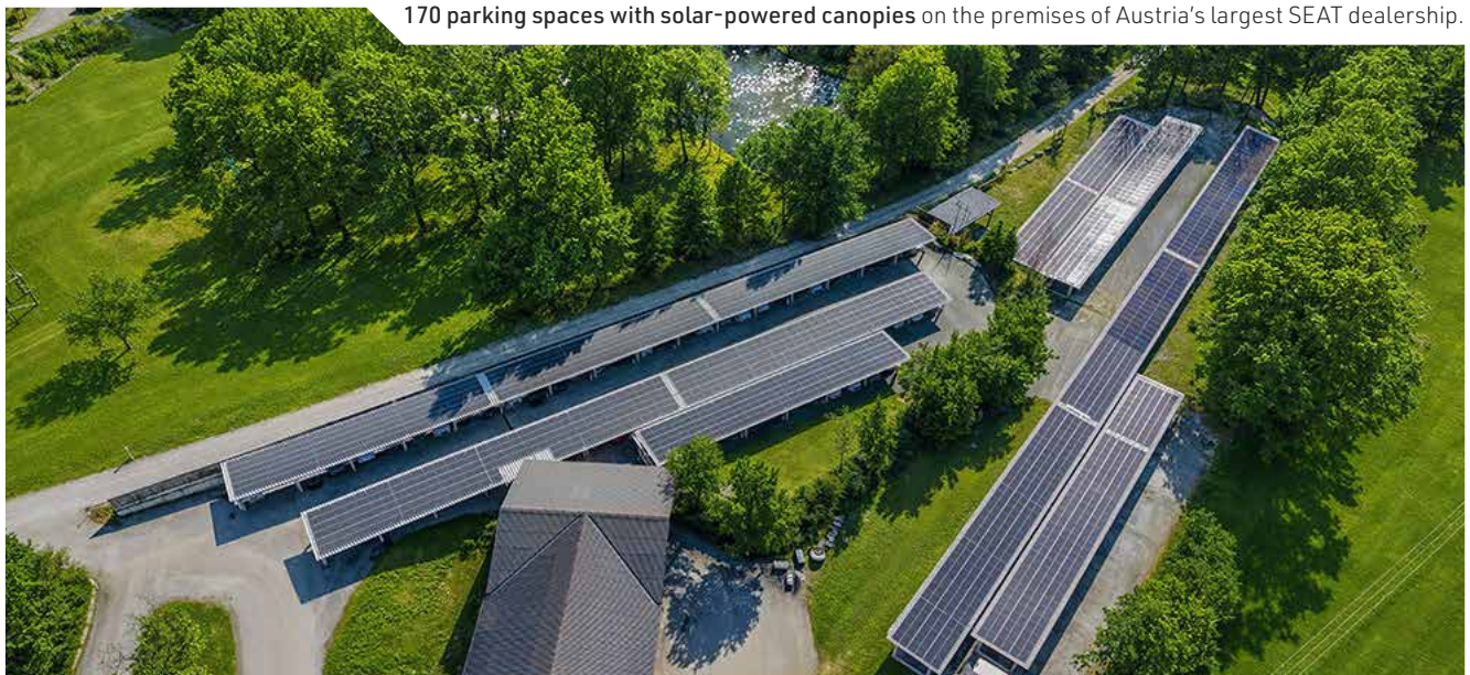
170 parking spaces with solar-powered canopies on the premises of Austria's largest SEAT dealership.
