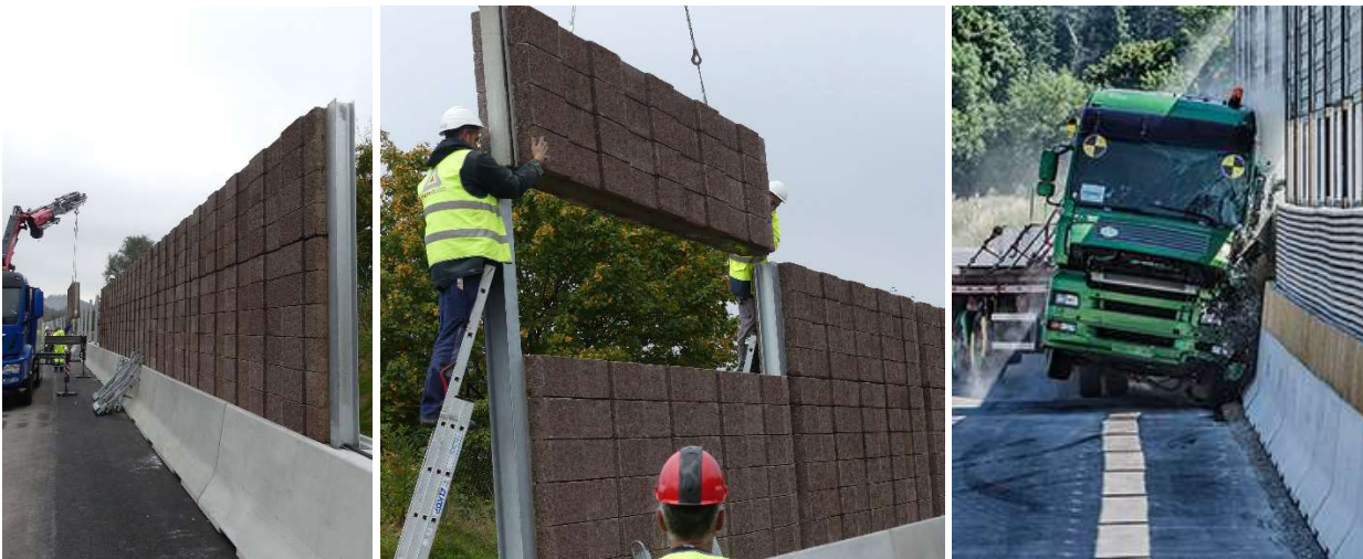
Left and center: PHONOBLOC® DB NBF installation along the A2 in Slovenia near Višnja Gora.
